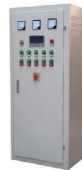
电控柜 Electric control cabinet
